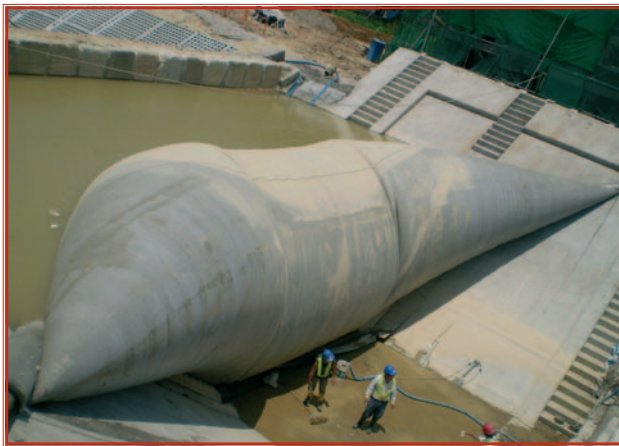
⬆️ 4.0m high Ma Wat rubber dam in Hong Kong.
