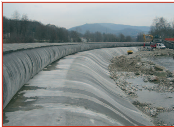
⚠ Chinese-made rubber dam on River Oglio in Italy.
