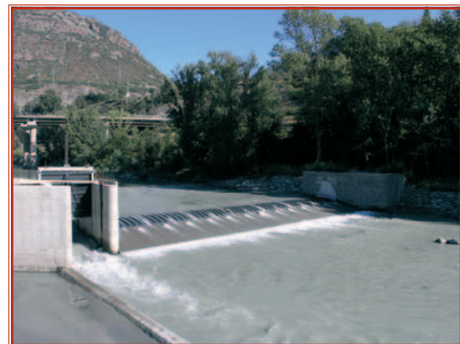
▲ Deflated spillway gate at HPP Pontey in Italy.
